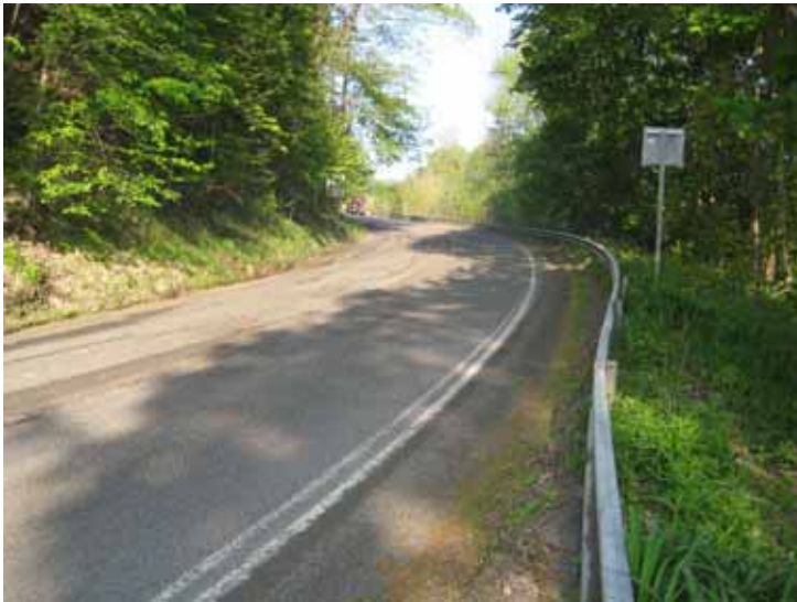
c. Route 39W Steep grades, Perrysburg, NY
